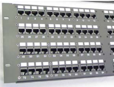
Network Patch Panel
